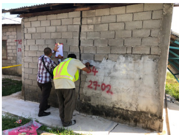
FIGURE 5. Measurement of a Cracked Wall
