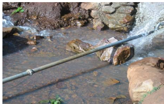
Fig.3. A pipe carries clean water from the source to a collecting point that is easily accessible for community members
