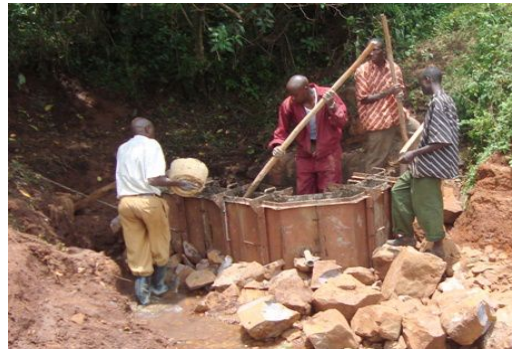
Fig.2. Construction of a barrier was the first step to providing clean water
